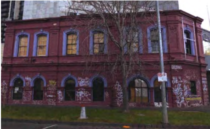
Figure 2 – Former Austral Otis Engineering Works office building, Kavanagh St frontage (proposed to be Significant under Amendment C305) – Source: Trethowan Architecture
